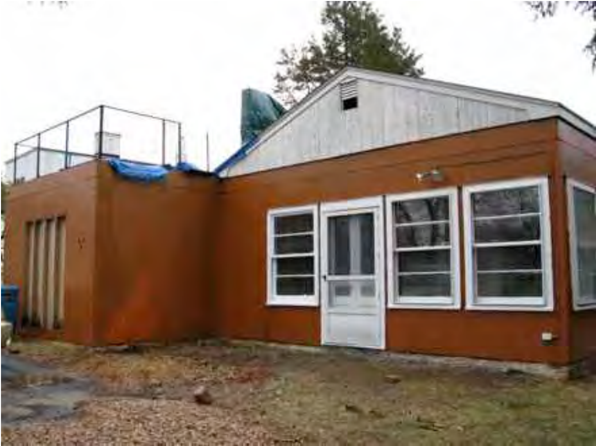
The steel house after Yankee Fiber Control had abated the peeling lead-based paint and applied Prax-Ten Penetrant to bare steel surfaces in April 2009 (author photo)
