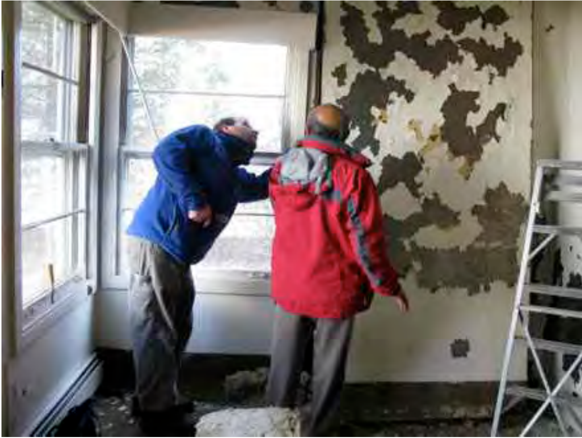
Metals conservator Adam Jenkins (left) and architect Barun Basu examine an interior wall panel at the steel house in early 2008 (author photo)
