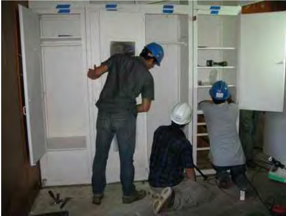
Workers from Milner + Carr Conservation disassemble the original built-in closets in a bedroom in late September 2011 (author photo)
