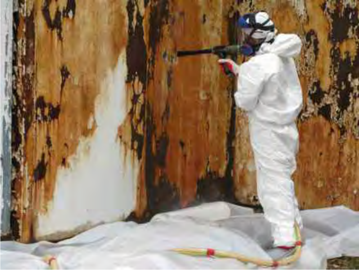
Workers from Yankee Fiber Control Inc. employ dry ice blasting to remediate lead-based paint at the steel house in March 2009 (author photo)
